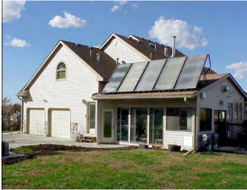
Solar Hot Water
