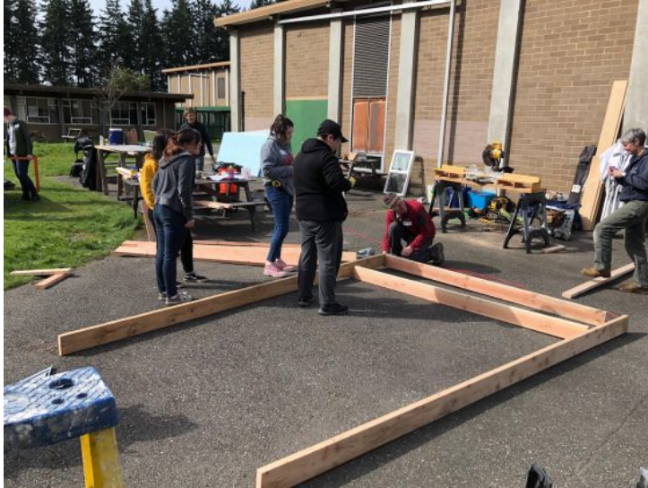
Scriber Lake High School students build the tiny house foundation. (Photo by Andrea Hillman)
