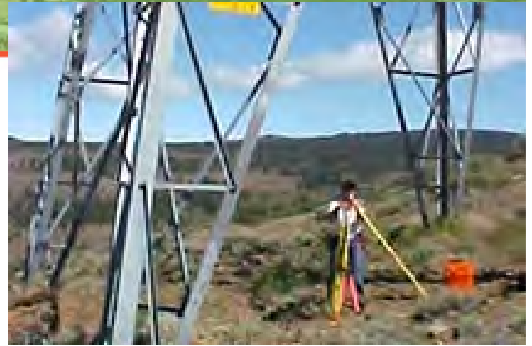
Schultz - Wautoma 500kV Transmission Line, Ellensburg, Washington
