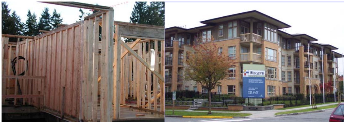
Figure 14 Application of Midply wall system in a four storey building, Vancouver, BC, Canada
