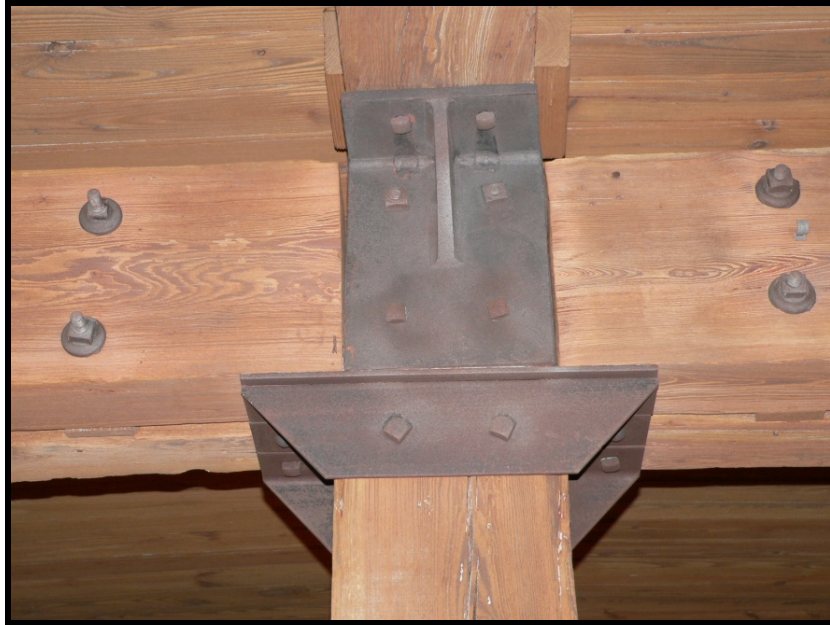
Beam-column connection with unknown capacity
