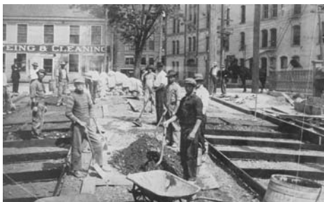
Figure 2 - A 1909 construction scene shows the first application of steel forms for street paving (From M.K. Hurd)
