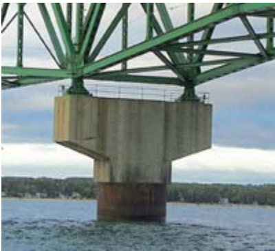
Figure 1: One of the thirty Mackinac Bridge piers investigated for scour assessment using OSI's 455kHz multibeam sonar.
