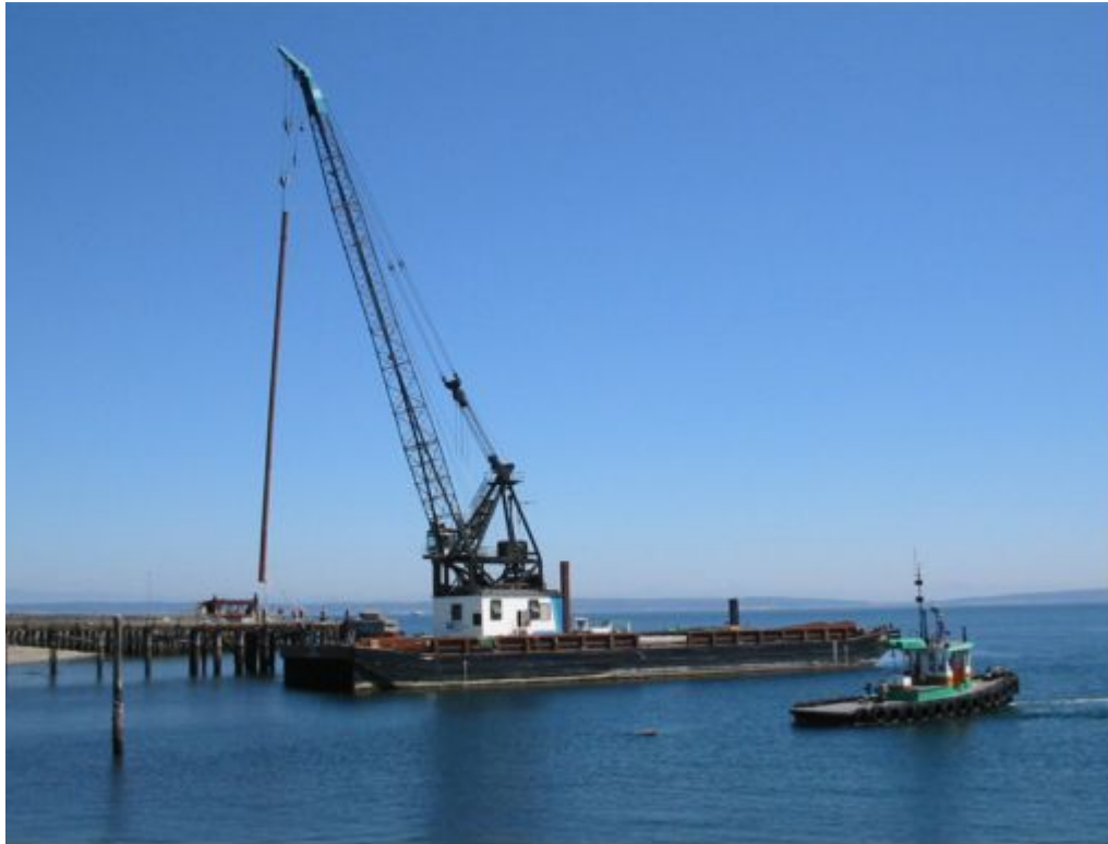
A 120-foot-long steel pile is swung into place at the end of the NWMC dock. Two test piles were driven in mid-August, providing dock engineers with information they needed to finalize construction plans.
