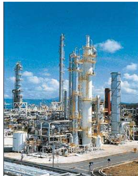
Figure 4: An example of an existing 200 ton/day chemical solvent capture plant in Malaysia (IPCC 2005)
