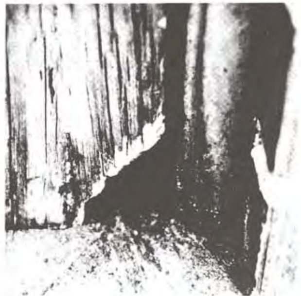
FIGURE 15. Rat gnawing in corner of wooden door.
