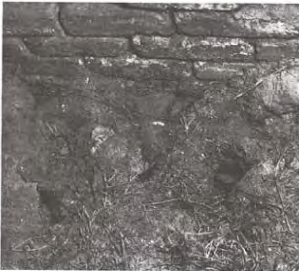
FIGURE 10. Norway rat burrows by a foundation wall.
