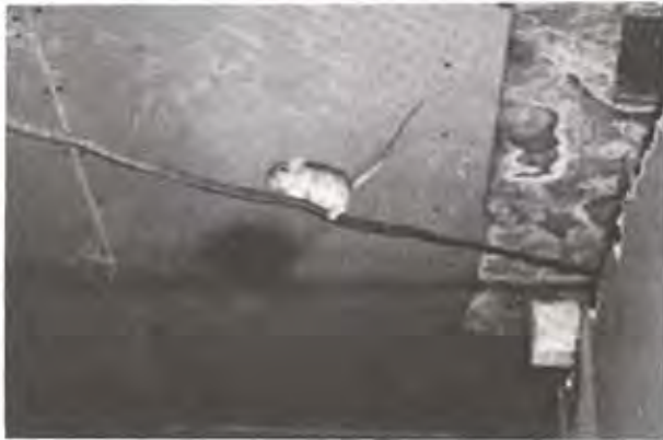
FIGURE 8. Roof rat running along cable.
