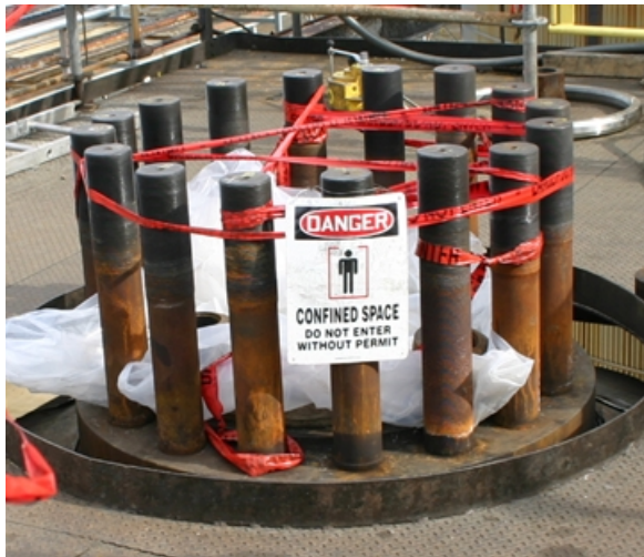
Figure 11. Confined space warning sign on the unsecured reactor manway after the incident.
