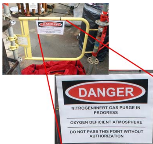
Figure 8. Nitrogen-purge controlled area barricade and warning installed on the R1 platform after the incident.
