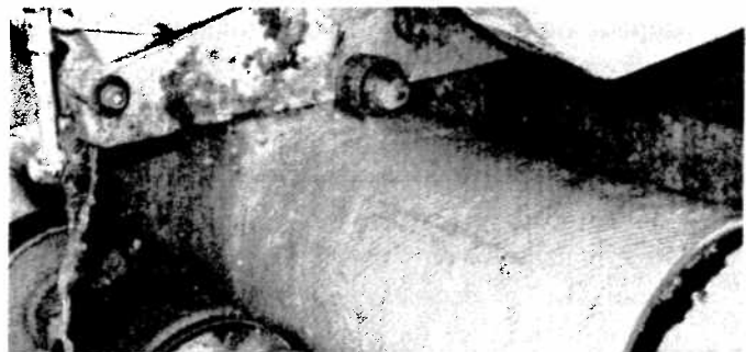
FIGURE 1-4. Water spray controls contaminants as pipe is cut. This is one of several control methods in addition to ventilation.
