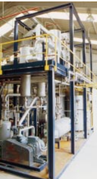
Figure 3: 200 kg/h Fast pyrolysis pilot plant at Union Fenosa, Spain
