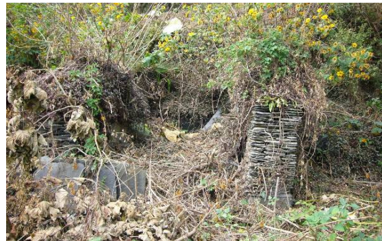
Type D : More than half of the walls have been demolished
