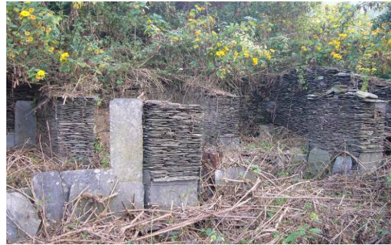
Type C: the walls of the house are partly demolished but keep a clear presence of plan
