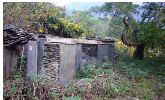
Type B: The walls and elevation are preserved well, only roof of the house is partly or completely collapsed
